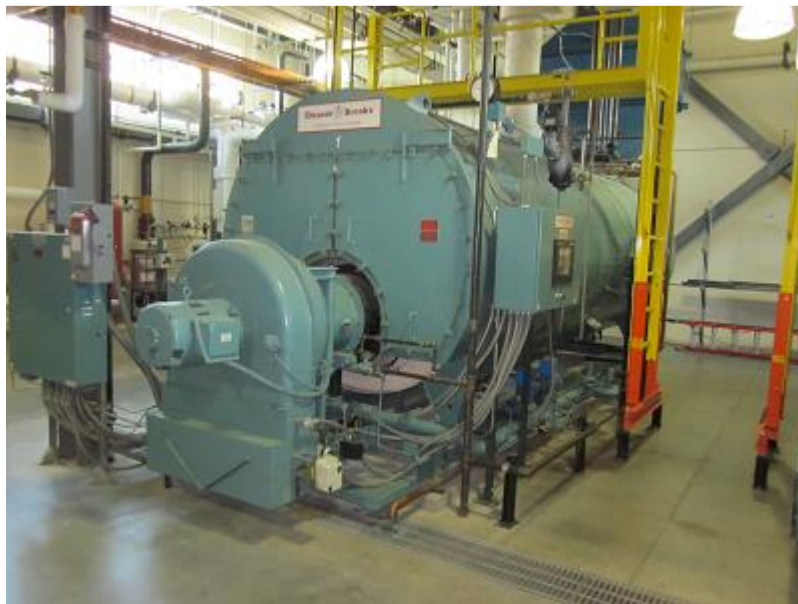
Typical steam boiler
