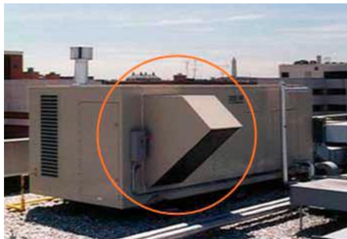
Outside air ductwork for air economizer – Source U.S. DOE
