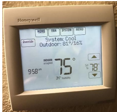
Programmable thermostat showing cooling setpoint
