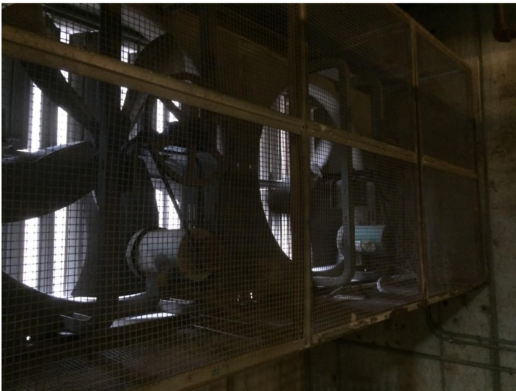
Garage exhaust fans
