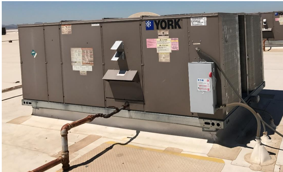
Typical packaged air conditioner
