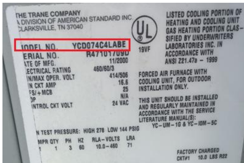
Nameplate data of a rooftop package unit
