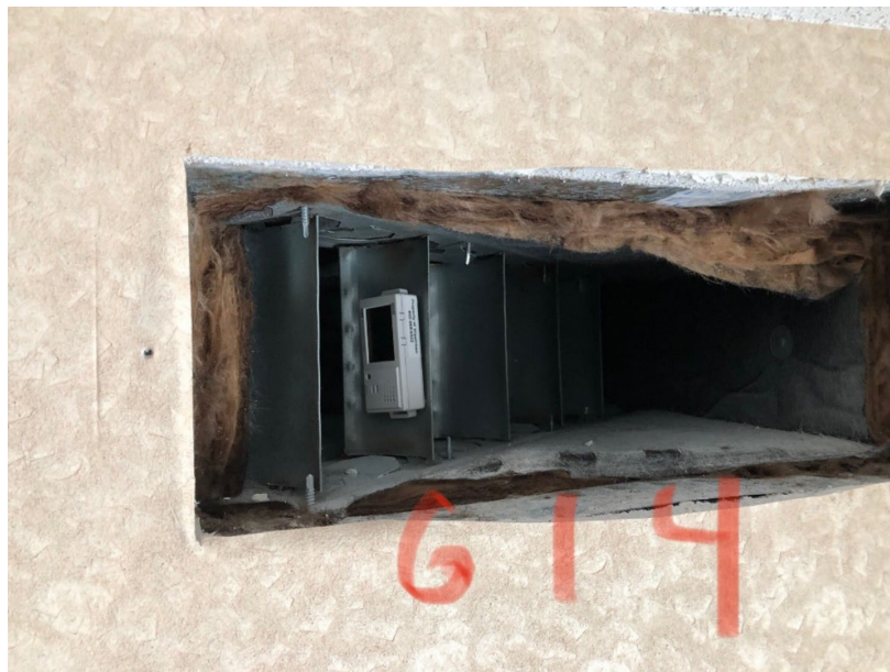
Figure 20: Sample Hobo temperature logger install in MAU supply duct at Drury.
