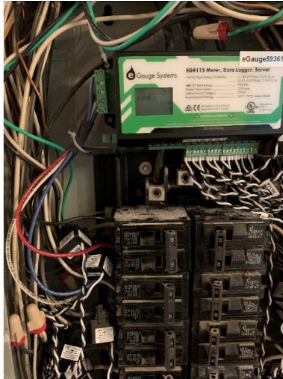
Figure 9: eGauge and current transducers installed in an electric panel.
