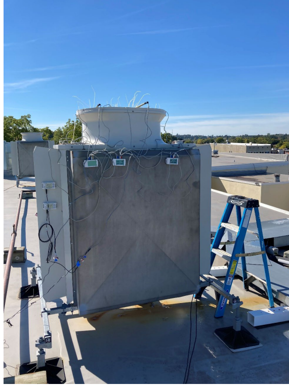
Figure 15: VRF-1 at Stafford's Perry hotel where outdoor airside measurements are being made.
