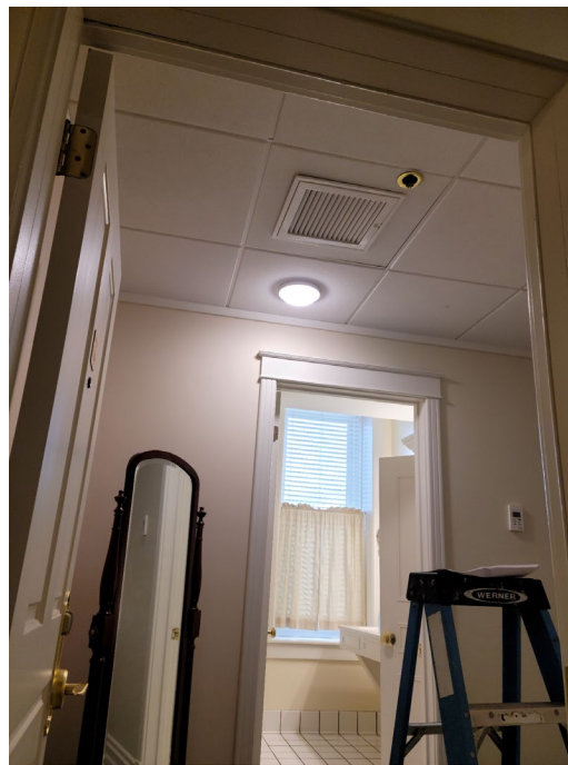
Figure 5: Supply air grille for indoor unit at Perry.
