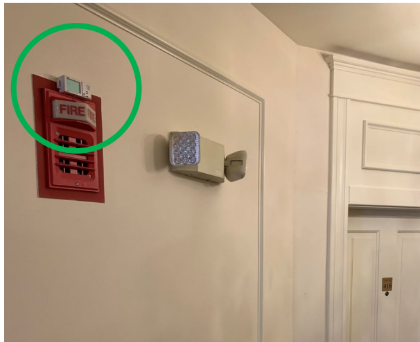
Figure 11: Typical hallway temperature logger installation.
