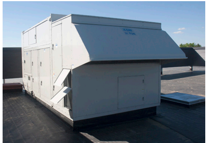
Figure 1: 749 University Row's dedicated outdoor air system
