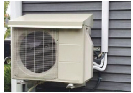
Figure 3 Proper placement: On brackets, insulated tubing, rigid line cover and drip cap.
