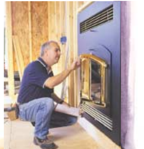
Joe Nagan inspects a fireplace in a home under construction. He’s checking for proper installation, proper ventilation, and compatibility with other equipment in the house.
