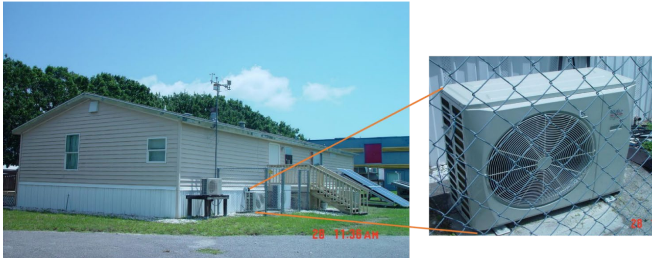
Figure 28. Picture of FSEC MH lab and the heat pump's outdoor unit
