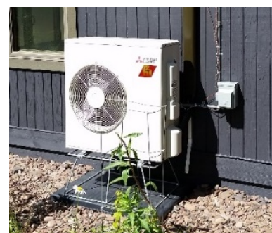
Figure 20: Photo of an ASHP
