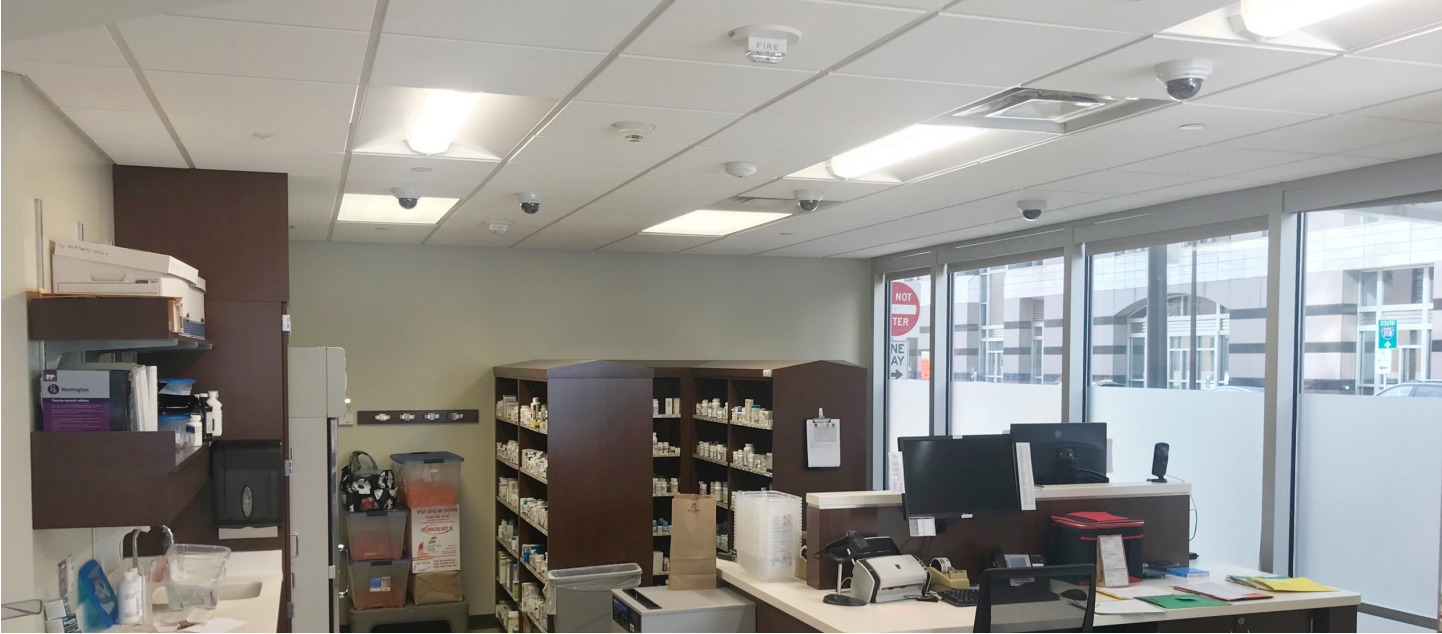
Controls are particularly impactful in the pharmacy, where light levels (and therefore base energy usage) are higher.
