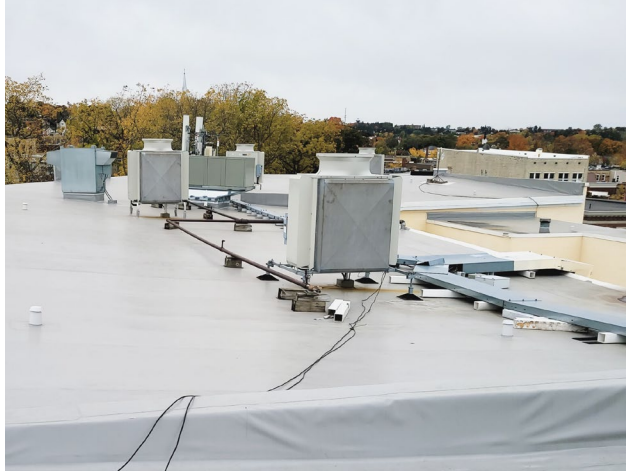
Figure 4: VRF units on the roof at Perry.
