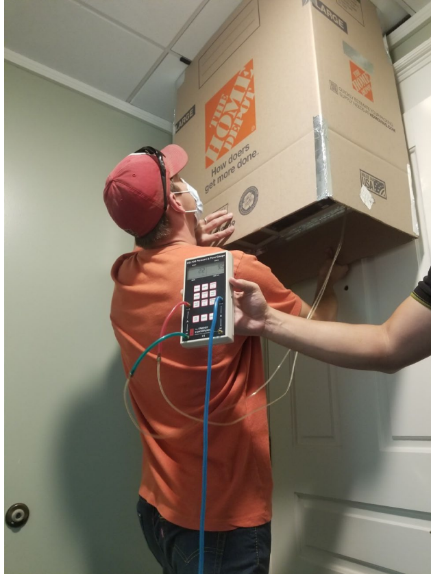
Figure 14: Making a flow measurement with the TrueFlow.
